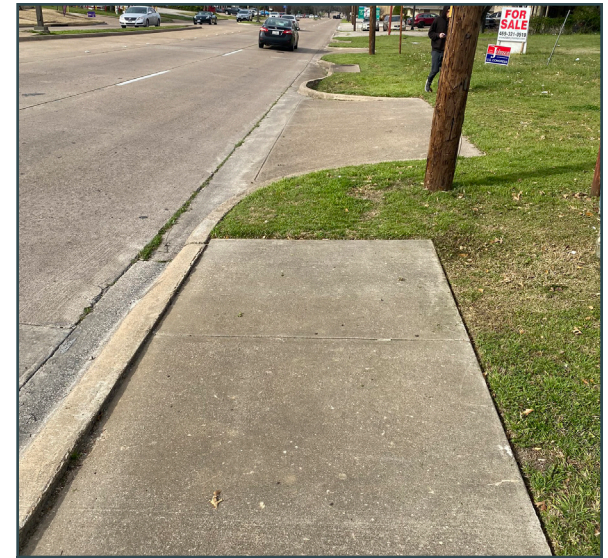
Sidewalk abruptly ends
