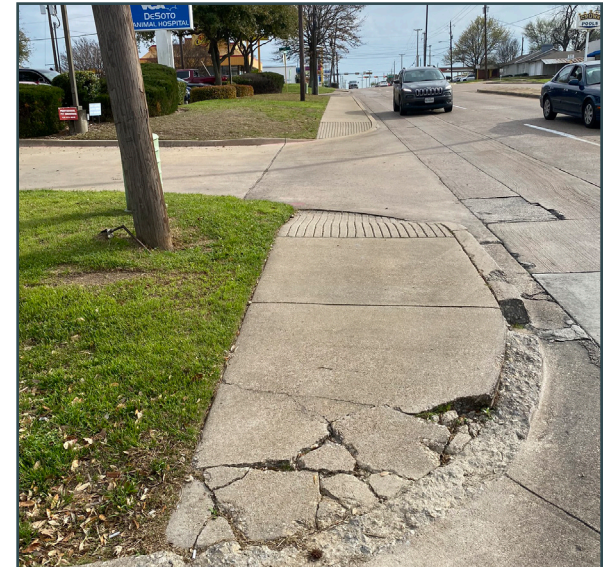
ADA accessibility issues exist
